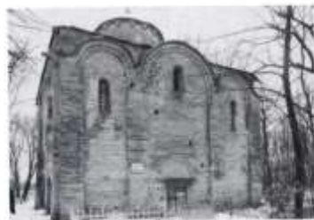
Figure 38. Church of Sts. Peter and Paul on Sinichia Hill, Novgorod. 1185-92. Southeast view. (N 18-20)
